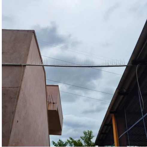
Protection of newly repaired security infrastructure to prevent future damage caused by forest monkeys. Bethel Orphanage
