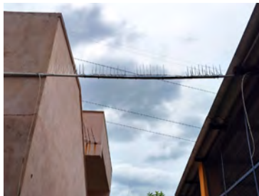
NOTE The spikes to deter future monkey damage.
